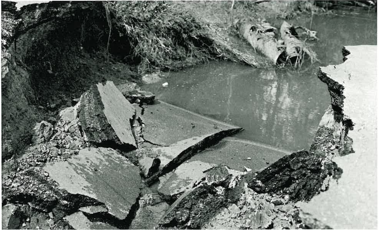
Washed out section of Highway 7 in Dallas County
