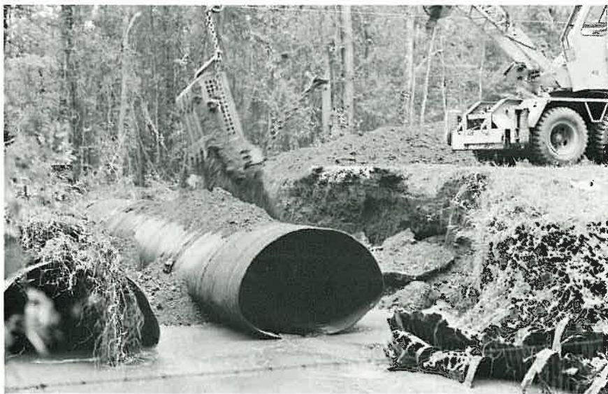
Once the new pipe was in place, workers began filling in the roadway section
