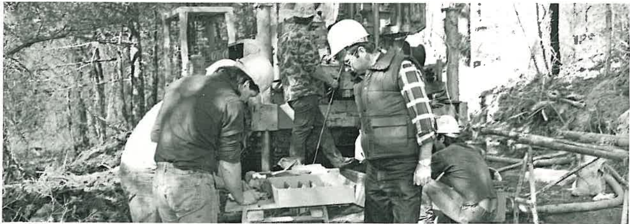
John Annable, right, checks out soil samples as they are logged by Steve Faulkner
